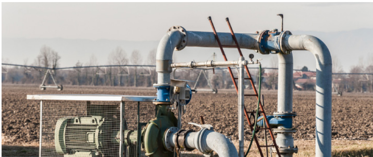
Electric motor irrigation system
