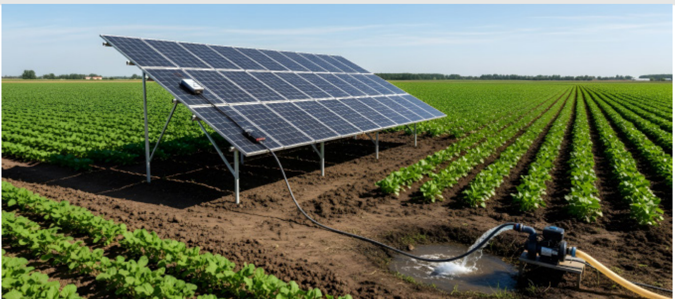
Solar Energy Irrigation System
